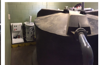
The Sodium hypochlorite storage tank
