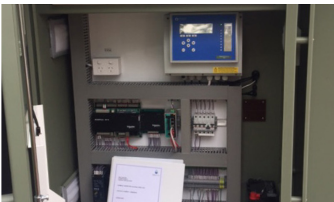
Electrical Panel housed within cabinet
