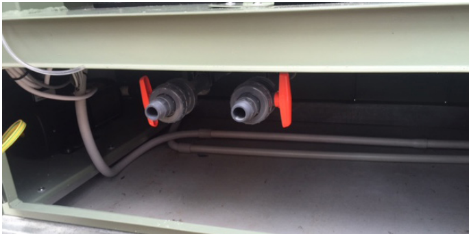
Drain taps from the bund
